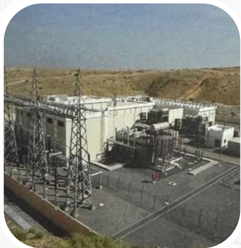
Oman Electricity Transmission Company Replacement of sensing components in fire equipment, smoke and heat detectors
