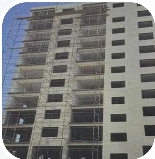
Al-Khairat School Endowment Building for Quran Memorization (Al-Ma'abila) Installation of new fire alarm system, fire fighting system and LPG connections
